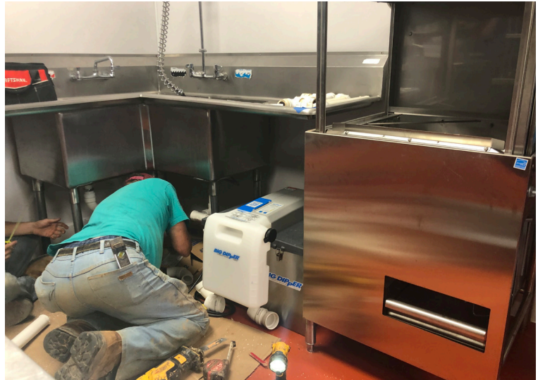
Plumbers had to fit the Big Dipper W-250-IS in Hamilton's Steakhouse in a tight space in the kitchen, between the prewash sink basin and dishwasher. They got the job done in under an hour.
