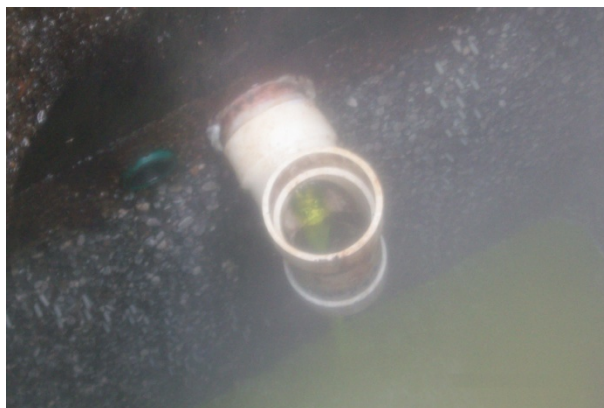
Dye Observed in Inlet of Concrete Grease Interceptor
