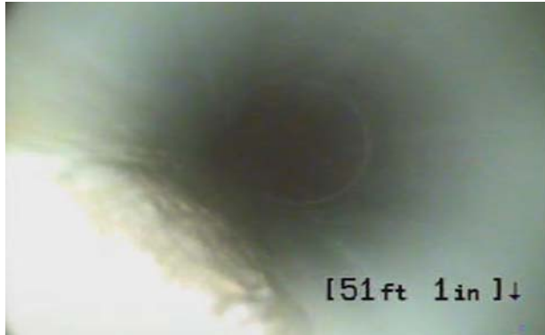
Private Sewer 51'1" Downstream of Concrete Grease Interceptor Immediately After Cleaning on 12/14/2011 4
