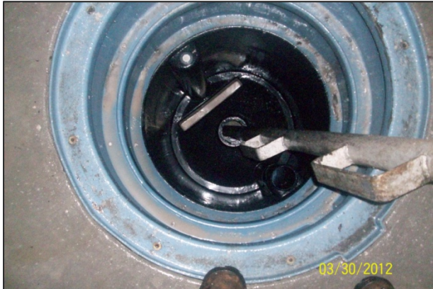
Interior of the Trapzilla® Immediately After Pumping on 3/30/2012
