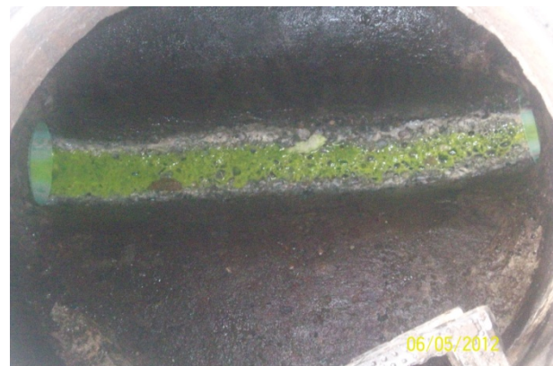
Dye Observed in Downstream Manhole of Private Sewer Line
