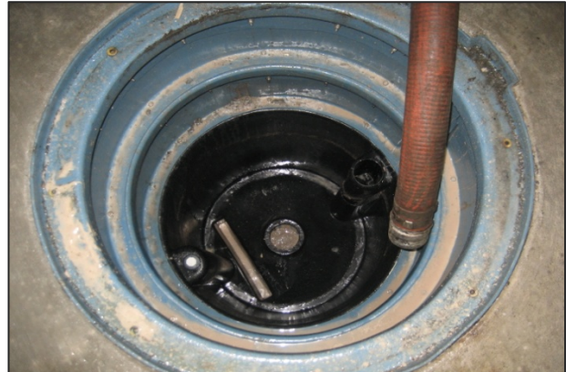
Interior of the Trapzilla® Immediately After Pumping on 5/1/2012
