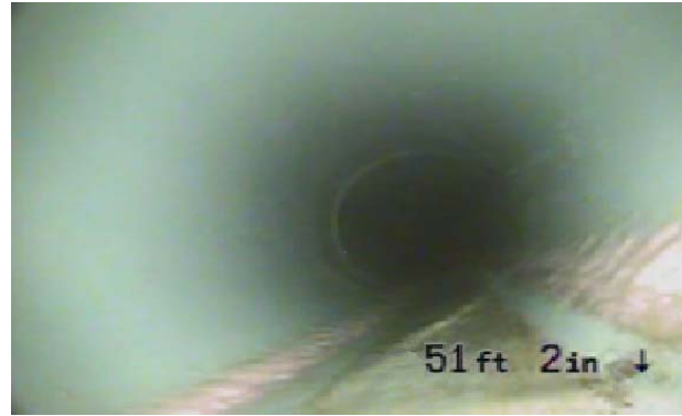
Private Sewer 51'2" Downstream of Concrete Grease Interceptor Two Weeks After Cleaning on 12/28/2011
