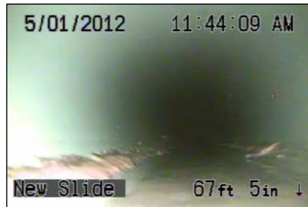
Private Sewer 67' 5" Downstream of Trapzilla® Two Months After Installation and Cleaning on 5/1/2012
